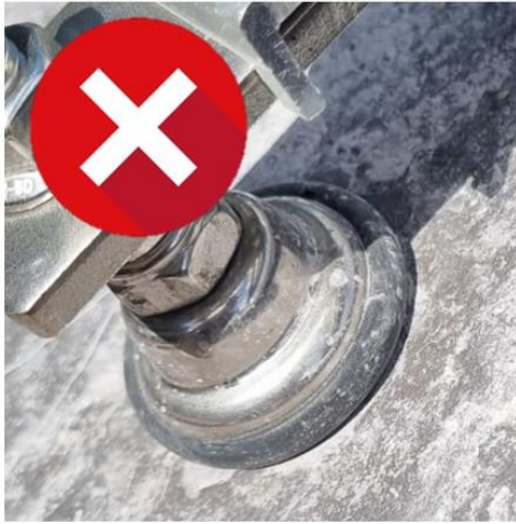
TOO COMPRESSED – Bulging outside the cap
