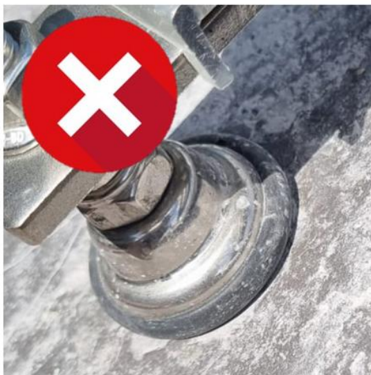
TOO COMPRESSED – Bulging outside the cap
