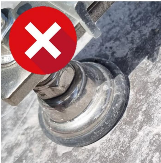
TOO COMPRESSED – Bulging outside the cap
